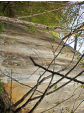
ひび割れ補修前
